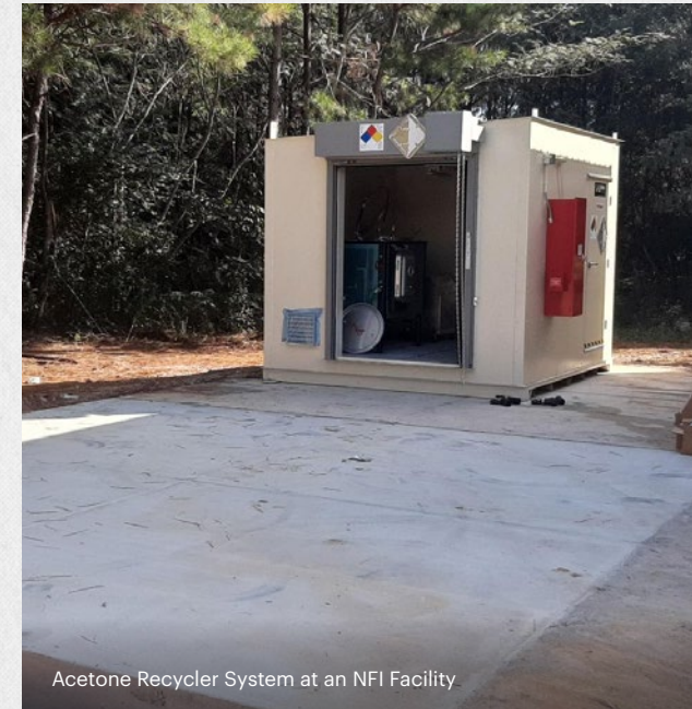
Acetone Recycler System at an NFI Facility
